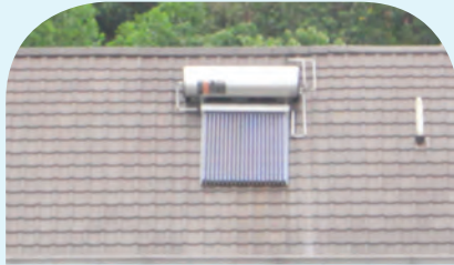
Panel solar ba perabung
