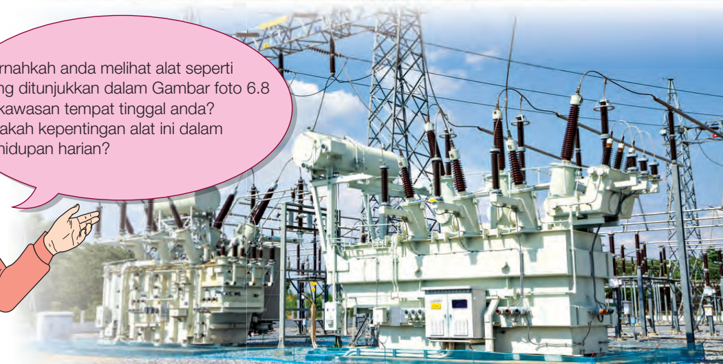
Gambar foto 6.8 Transformer
