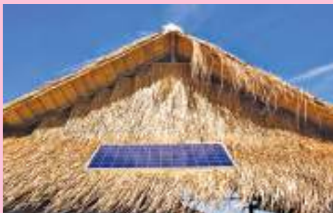
Roof with solar cells
