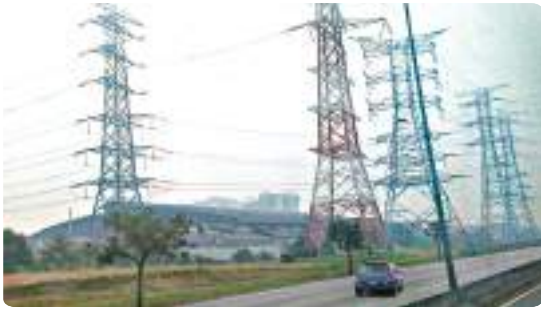
500 kV alternating current transmission cables along the North-South Highway.
