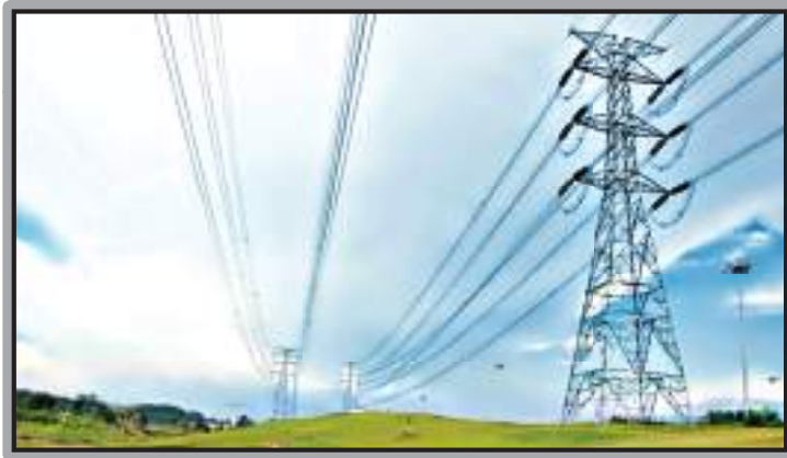
Photograph 6.10 Transmission cables on the National Grid Network pylons
