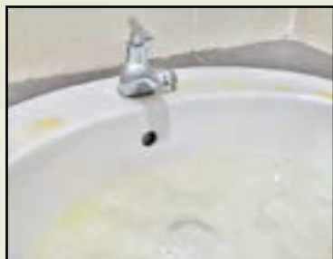
4. Clogged kitchen or bathroom drains
